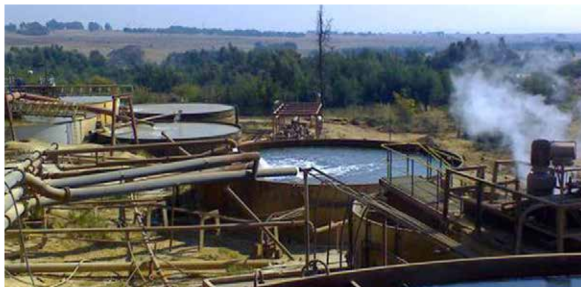
Sunderland wastewater treatment plant in South Africa emitting gases into the atmosphere
